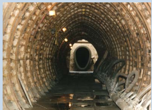
Figure 6: Ground water reserves in the gallery
